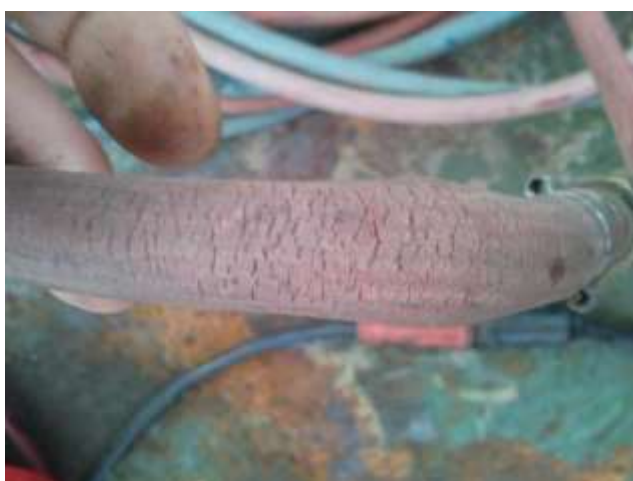
Left: work-hardened and perished hoses
